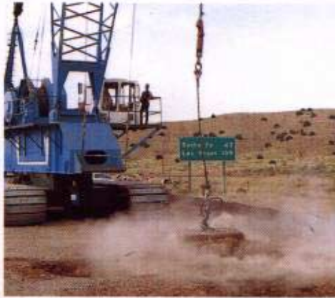
Collapsible soils, Albuquerque, New Mexico
