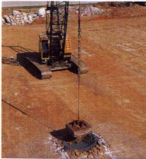
Dynamic Replacement showing backfilling craters with stone prior to repounding. Questionable silty fill, Winchester, Virginia
